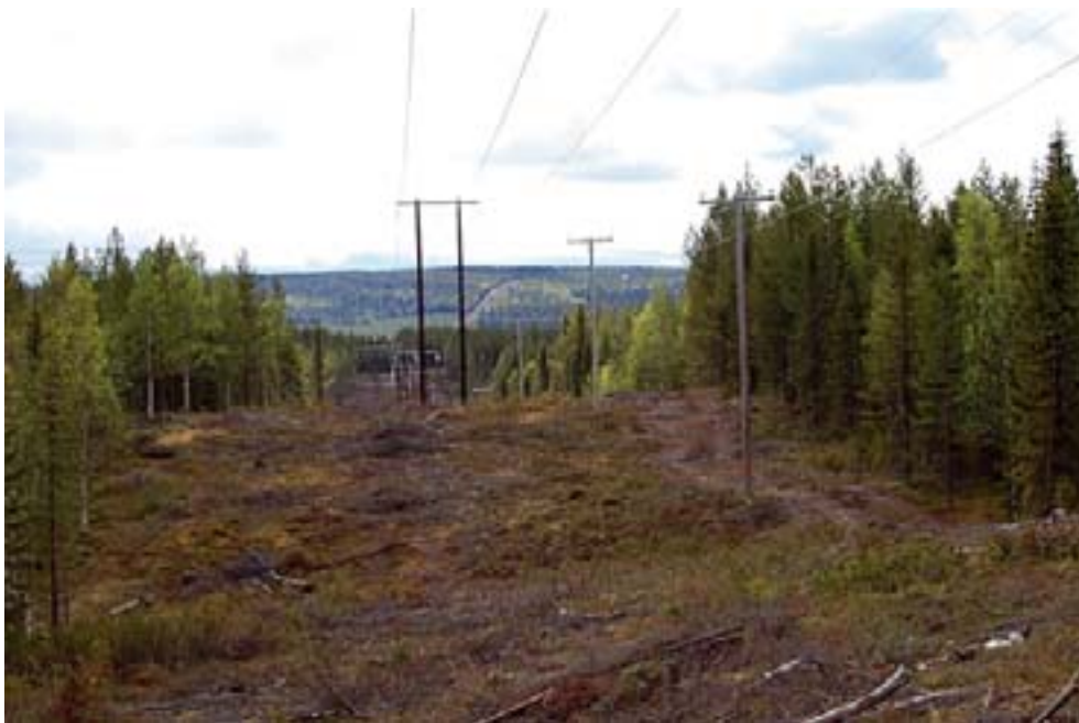
New power line at Jokkmokkliden wind farm in northern Sweden. Another new power line, for Storliden wind farm, is visible in the background. Photo: Anna Skarin.
