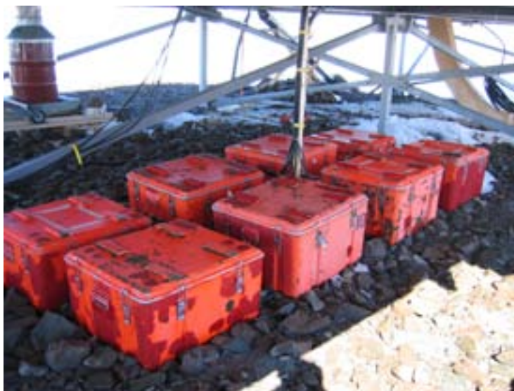
Figure 18: The battery bank at Wasa station.
